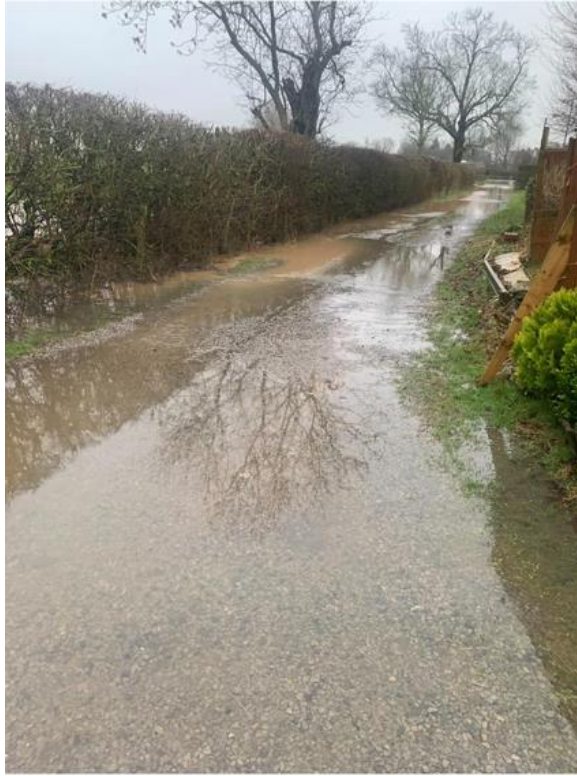
Photograph One- Flooding damage
